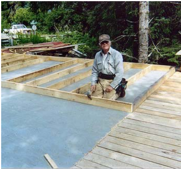
Joe as he starts to build the frame for a wall on the new shop.
