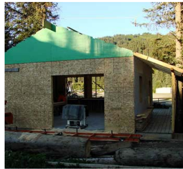
The shop with walls, just before the roof is put on. Joe also built his own trusses.
