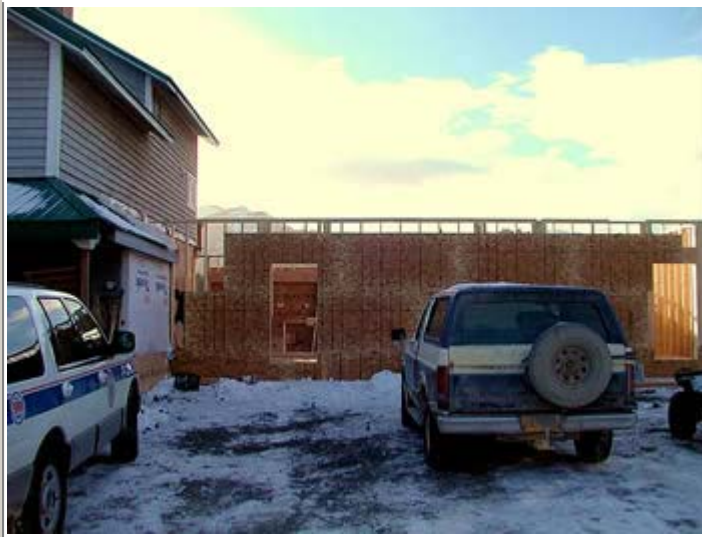
Tide Pool Restaurant is in front of the Police Car, the new extension view is facing the street.
