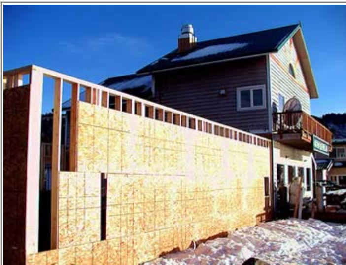
View from the harbor side of the Tide Pool's expansion project. Windows are not cut out yet.
