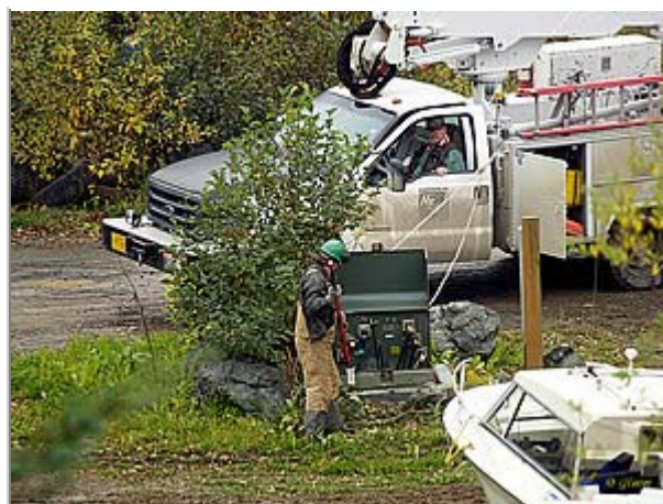
Before the cable can be repaired, switches like this unit must be tripped in order to kill the power to the damaged part of the grid.
